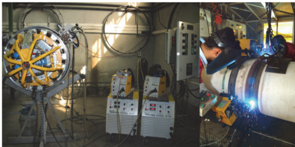
Fig. 5. Automatic pipe line welding system in the experiments (made by Novin Sazan Co.)
